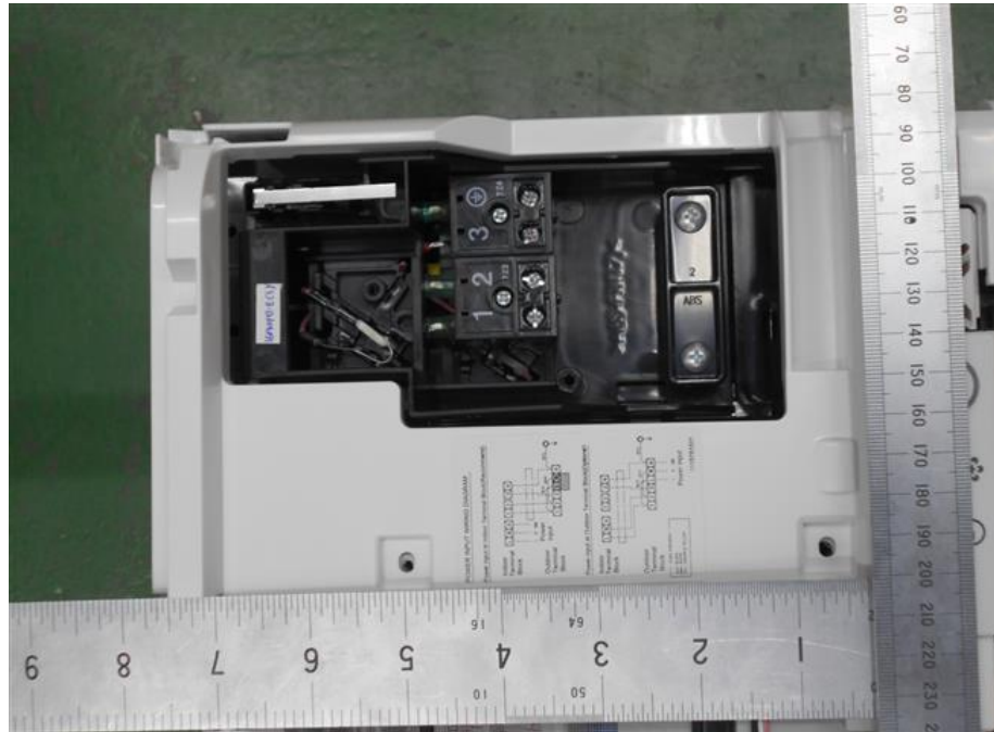
31. RAS-M10PKVPG-E, Terminal supply, interconnecting terminal, wiring diagram, micro switch and cord anchorage
